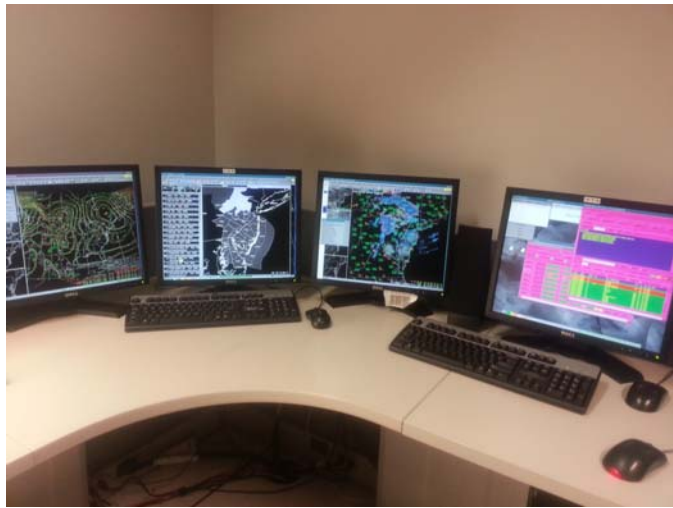
Here is another look at the consoles
