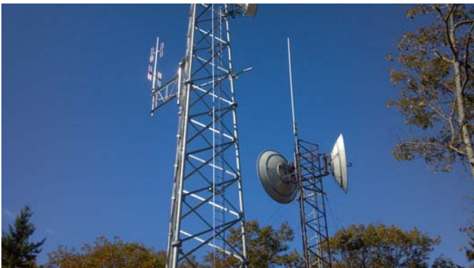
New site being installed as part of communications infrastructure upgrades, above and several pictures below:
